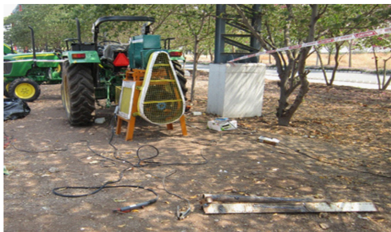
Fig. 5: PTO driven generator with DC load
