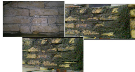
Fig. 7: Bigger cracks initially originate from the lower two sample ends
