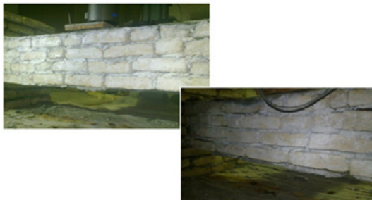
Fig. 6 : The failure of mortar and bricks at the lowest sample parts
