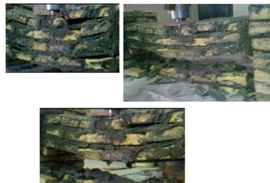
Fig. 9: Cracking and detachment of material in the reinforced beam
