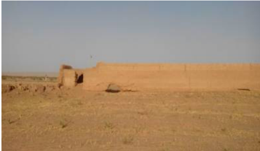
Fig. 5: Erosion of north wall of the building by the wind (writer, 2014)
