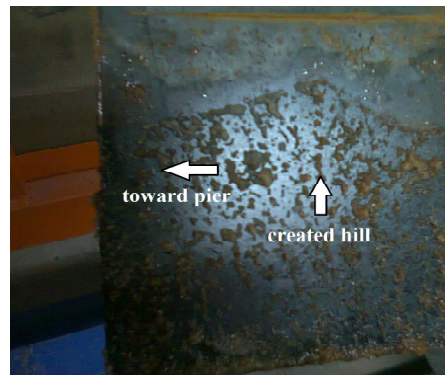
Fig. 9: Longitudinal scour and deposition on the face of middle plate
