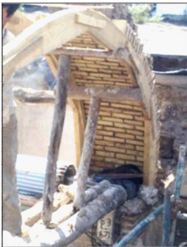
Fig. 9: Assembly of two pieces of wooden templates and the way wooden holder is installed for more stability. Dokhan-Caravansary, Zanjan
