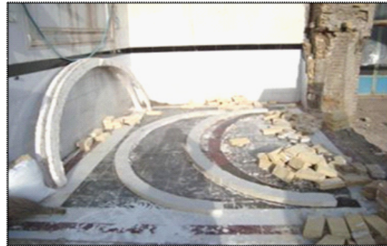
Fig. 4: The arrangement of the bricks in hemicycle form and filling it with gypsum slurry in order to create a semi.Tavizeh in sharp-chafd form.
