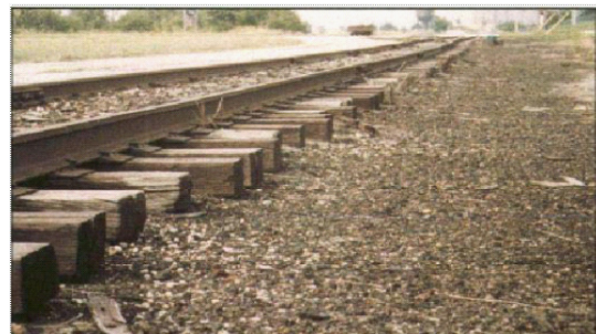
Fig. 4: Ballast at the shoulder and the inadequacy
