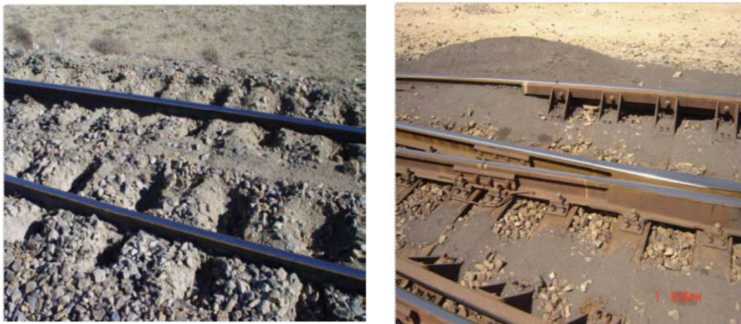
Fig. 2: An example of failure ballast
